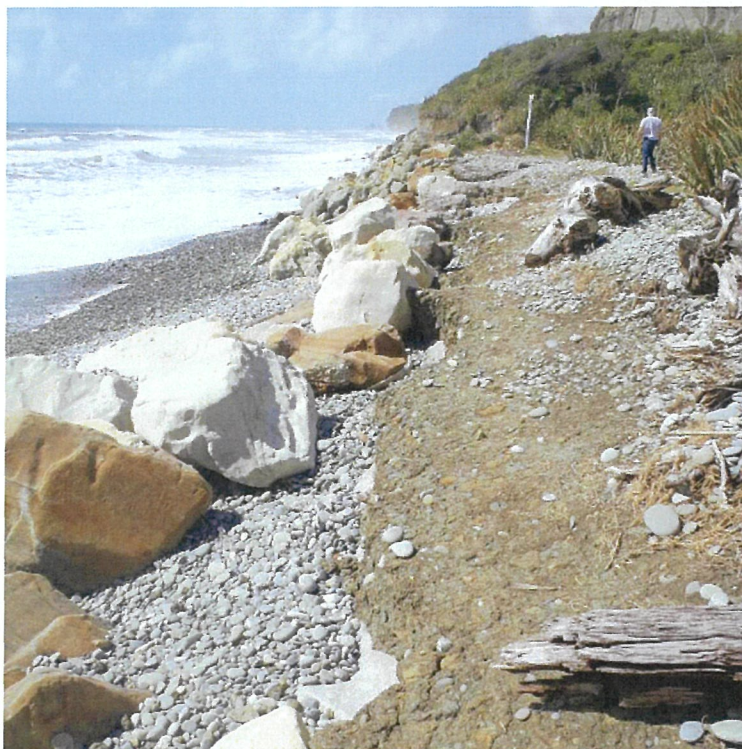
Figure 3-5: Current condition (21 November 2016) of the northern end of the rock revetment. [Credit: M. M. Allis].
