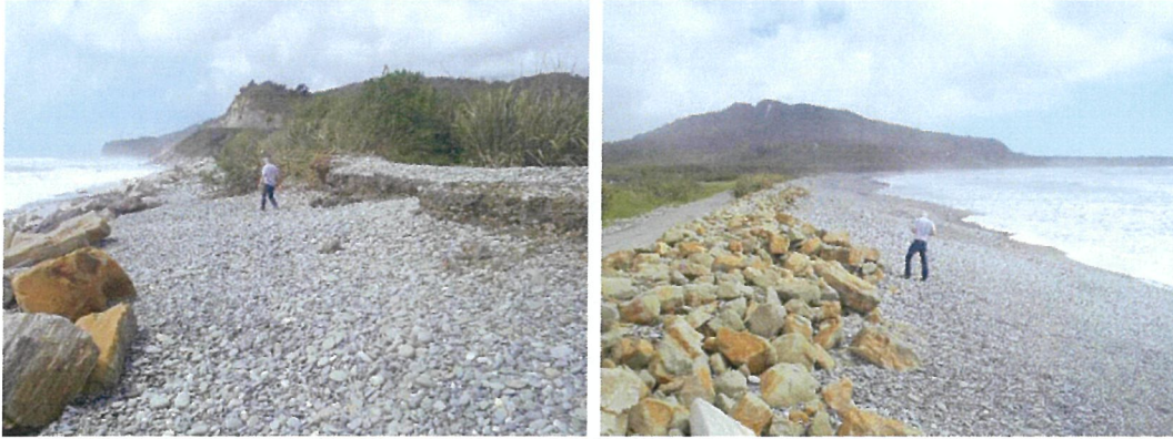
Figure 3-3: Continued erosion behind the rock revetment along the former Beach Rd between Morpeth St and Holland St (left) and recent protection works alongside Beach Rd south from Statham St (Right). Left: note former Beach Rd tar seal and basecourse layers at right of image. [Credit: M. Allis].
